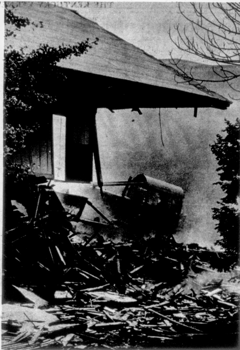
Bulldozers moved in on Splinter Hall Aug. 17 to do what a severe fire had not done. Arson is believed to be the cause of the fire.
