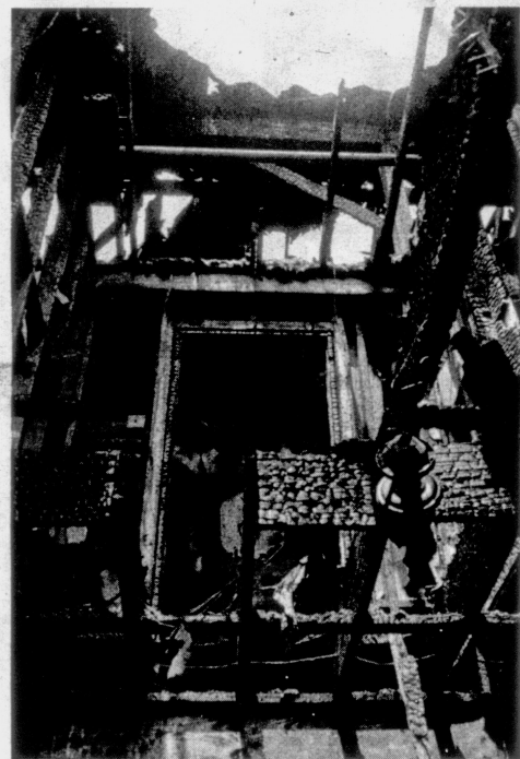
The lounge area in the center of Splinter Hall (above) is thought to be the point where the fire started. Although the outside of the building was undamaged, the interior was gutted, making repair of the frame structure virtually impossible. This photo is from the files of the Safety and Security Department.
