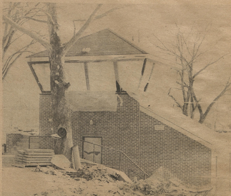
The new entry station at KCIW is nearing completion. The new facility, on which construction was begun last summer, will house visitors' restrooms and lockers and a strip-search room, in addition to its function as an entry station.
