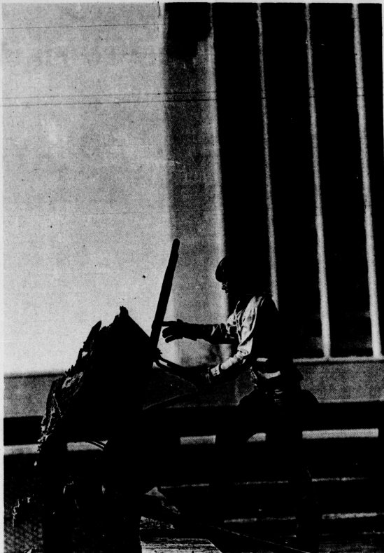
That last step... Charles Brotherton, UK employe, helps replace a weather-damaged roof on the Fine Arts Building. Most of the roofing landed in a dump truck parked below.
