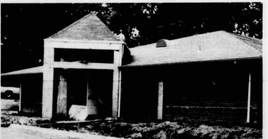
Sit located on construction, Kinder-Care Learning Center, UK's first full-time day care, is located on the corner of Columbia and Woodland Avenues.
