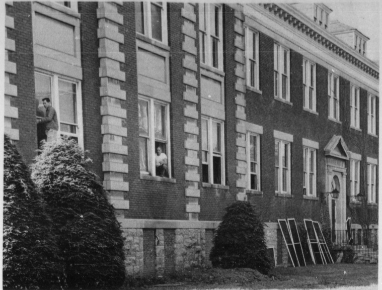
Renovation work has begun on Kastle and Pence halls. Construction is due completion by Aug. 1, with opening date set for Sept. 1.
