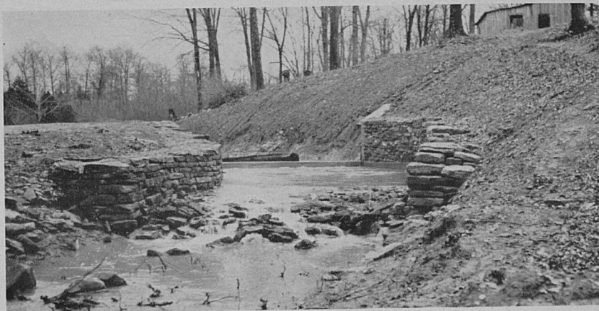
FIGURE 10. A spillway of concrete and loose stone.
