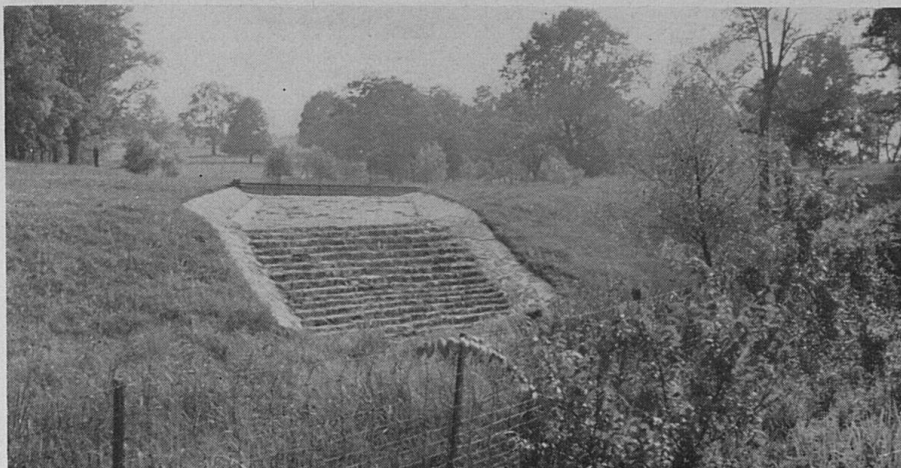
FIGURE 5. A farm reservoir with a masonry spillway directly over an earth dam, as a feature in landscaping.
