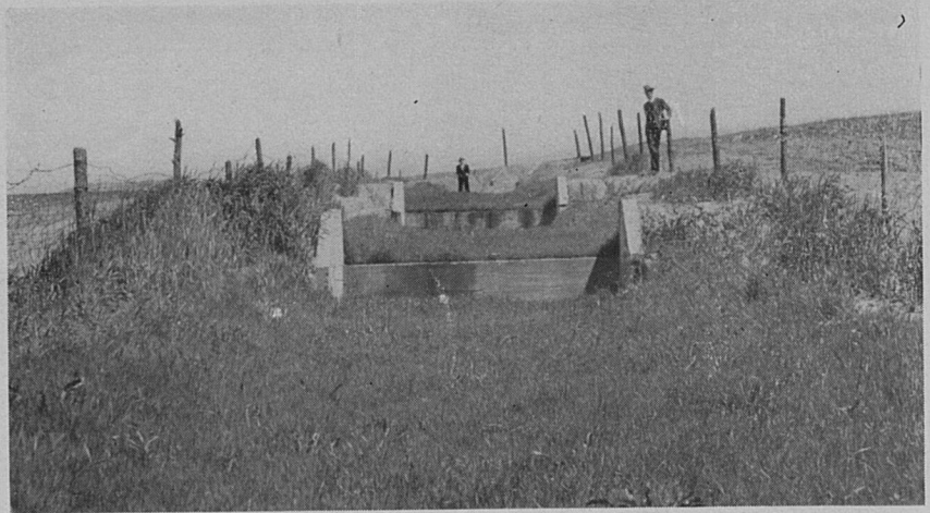
FIGURE 13. Spillway of large reservoir, protected from erosion by concrete check dams and vegetation.
