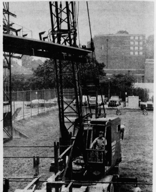
A construction worker maneuvers a crane to remove benches from Stoll Field to respective positions in the end zones of the new Commonwealth Stadium. (Kernel photo by Brian Harrigan)
