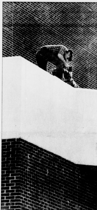
Drill bit Two Physical Plant workers take advantage of yesterday's nice weather to make repairs on the Center for the Arts roof.
