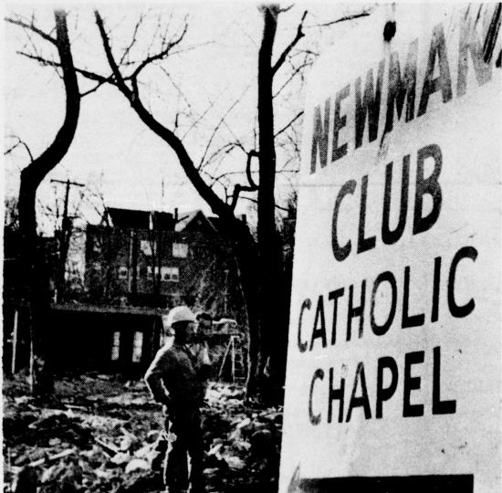
A forlorn sign points to rubble as these two workmen take a break from their dreary winter's work of tearing down the Newman Center. (Staff Photo by Ann Firesheets).
