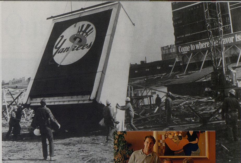
The first phase of the major reconstruction program for Yankee Stadium included lowering the Yankee logo from the old scoreboard. Invirex Demolition Inc., completed this job of "selective removal" of structural elements five weeks ahead of schedule.
