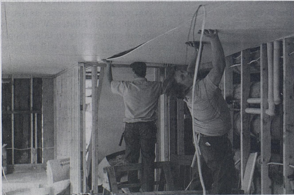
FNS maintenance men Joe Hacker (left) and Kenny Bowling at work renovating the old log barn at Wendover. The small apartment will be home to David Lee and Stacey Wilson.
