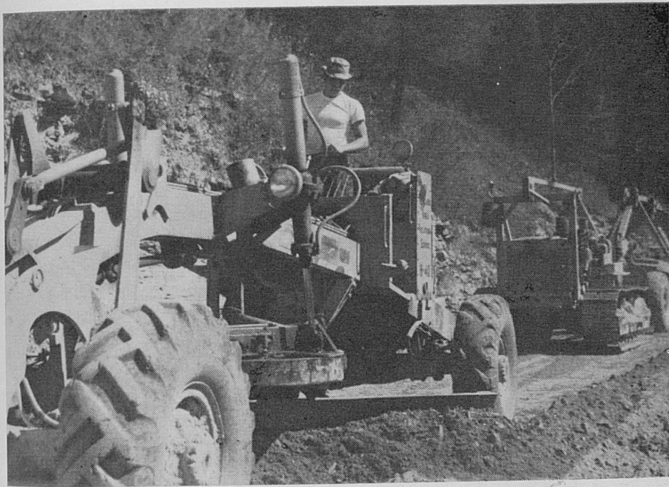
Industrial As Well As Residential Sites Are Enhanced by the Bulldozer's Blade
