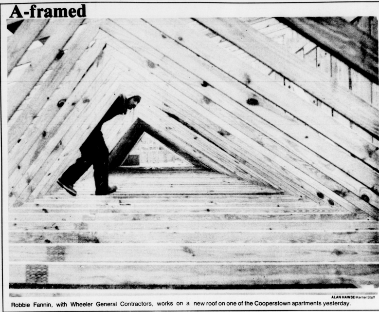
Robbie Fannin, with Wheeler General Contractors, works on a new roof on one of the Cooperstown apartments yesterday. ALAN HAWSE/Kentucky Kernel Staff
