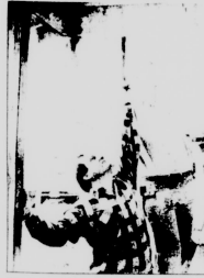
Home John, left, holds a section of sheetrock in place for Tony Deim to nail in place while working on the home of Matthew and Caille Clem on Hill Street. Members of the Hill Street Pentecostal Church of God have been working to improve living conditions for the couple for several weeks.
