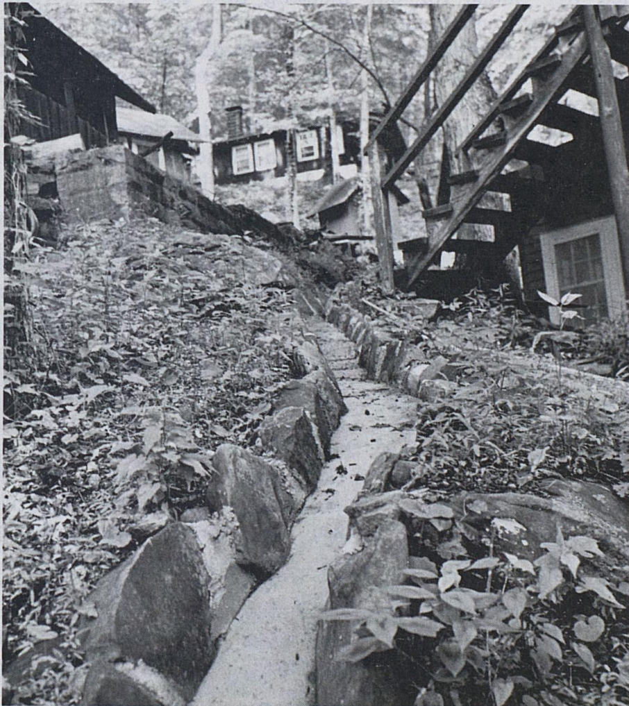
New drainage ditch at the Big House with the Upper Shelf in the background.
