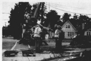
Arrow Electrical Contractors begin to replace the metal pole at the corner of High Street and Fontaine Road that holds the street signs and cross walk signals.
