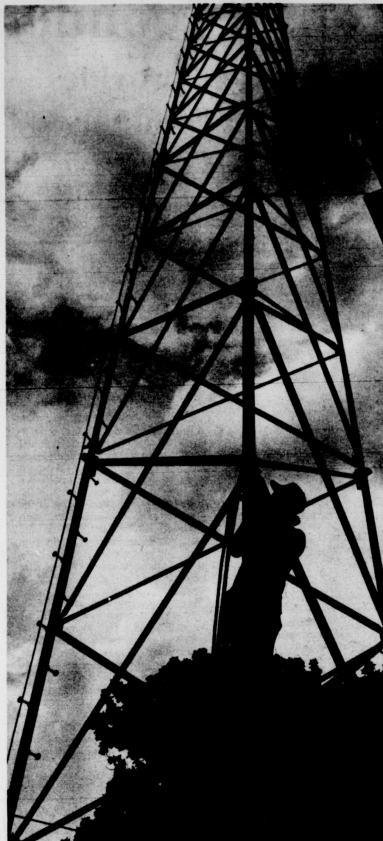
A worker climbs one of the six light towers installed this summer at Shively baseball field.
