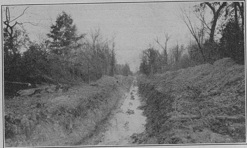
Drainage project in Hopkins County where 23 farmers raised $5,400 and re-established the Elk Creek drainage channel. The ditch is 2\frac{1}{3} miles long.
