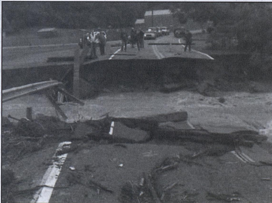
Hwy 421 - Flood Damage (photo courtesy of Katelyn Dykes)
