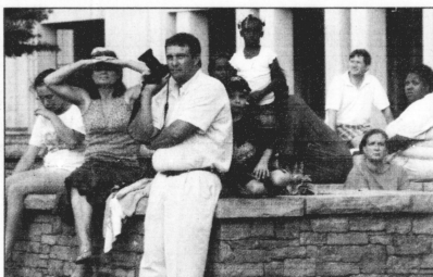
Sheila and Judson Ridgway of Lexington watch with their family as the Rite Aid Pharmacy Building on the corner of Limestone and Main Street is torn down yesterday evening.
