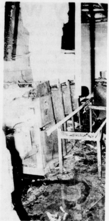
This is part of the equipment which was damaged when fire broke out in the Controller's Office in the Physical Plant on Wednesday. (Photo by James Coyle)
