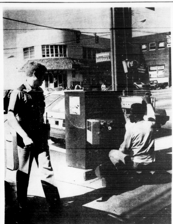
Lights out A Lexington police officer looks on as a repairman fixes a problem with the traffic lights on the corner of Limestone and the Avenue of Champions Friday afternoon.
