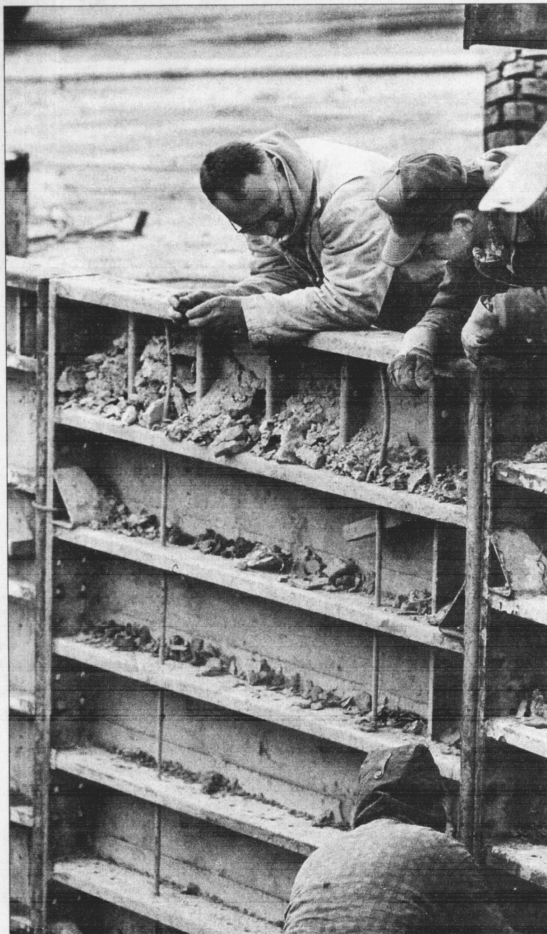
Congleton and Hacker Construction workers Steve Ritchey (left) and Lloyd Felty worked with Pete Fary (bottom) to put up a safety wall on North Campus.
