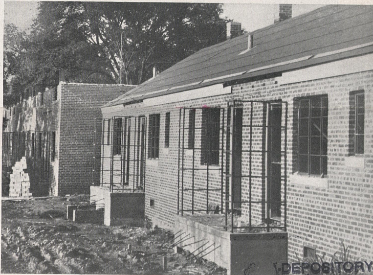
Elyton Village (860 units) is the first of Birmingham's three USHA-aided projects to open. It follows Smithfield Court (built by PWA Housing Division) as the second project for the city.
