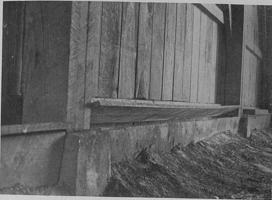
FIGURE 13. Inside view of bottom ventilators built on a dark fire-curing barn as shown in Figure 14, between the concrete blocks that support the barn posts. The middle door is shown partially open.
