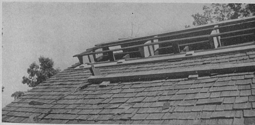
FIGURE 6. Ridge ventilator being constructed on wooden shingle roof according to Plan No. 1, Figure 7, page 12.
