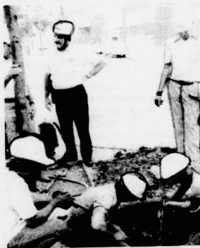
Several men try to plug a gas leak after a pipe was broken last night during construction on the Kincaid Tower site near the downtown area.
