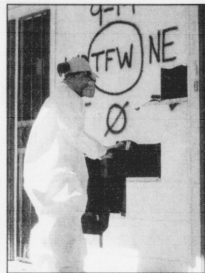
University of Detroit Mercy student Adrianna Hall, 19, from Warren, wears protective gear as she removes water-damaged siding from a flood-ravaged home in New Orleans on March 8.
