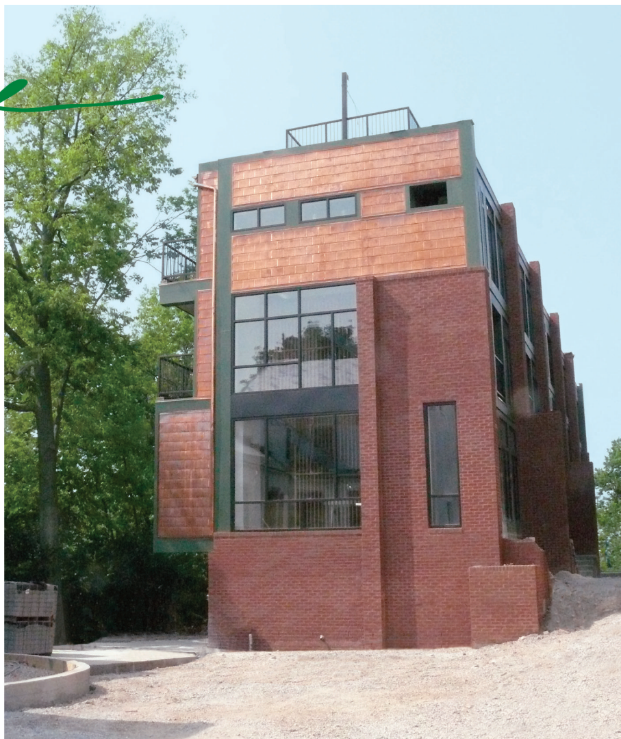
First phase while under construction and before any landscape or driveway improvements. Building exterior features brick veneer with copper shingles and downspouts.
