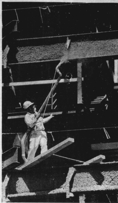
By J.D. VANHOESE/Kernell Staff Artful Dodger An employee of C.E. Pennington General Contractors of Lexington, coats the frame of the Second National Plaza currently under construction on Main Street downtown.
