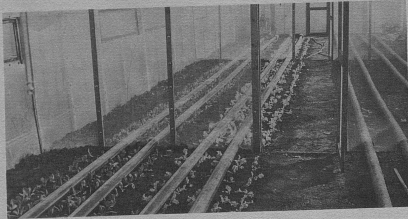
Fig. 2-- Black plastic tubes running through house from heating header. Partitions are for experimental tests.
