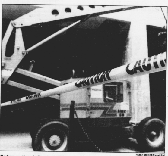
Workers sectioned off parts of White Hall Classroom Building to keep students away while the structure is hoisted, resurfaced and painted.
