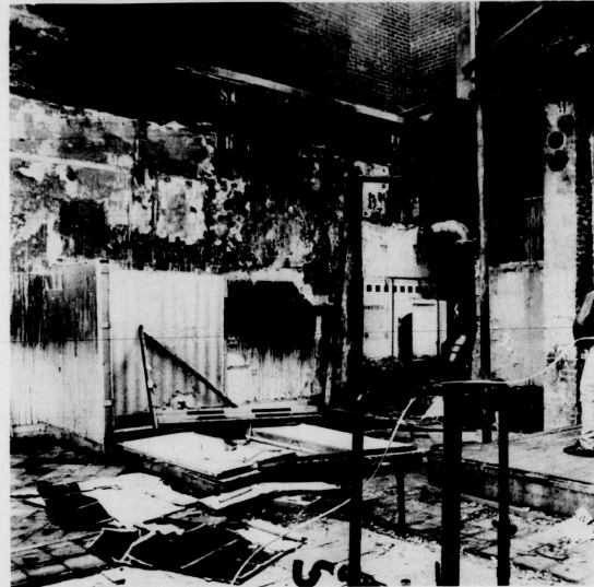
The fire at the Kentucky Theatre burned the manager's office and the restrooms. Because of fire damage, which could still mean extensive repairs.
