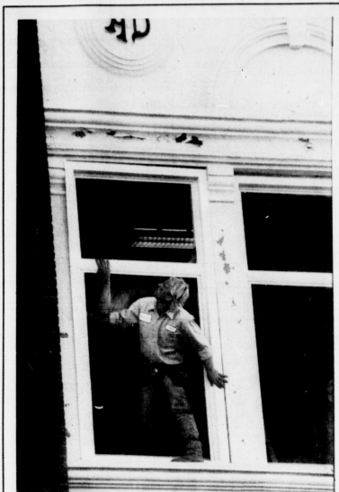
ON A LEDGE: Primax window installer Gary Smith steps out on the ledge while Dennis Sanders holds a new window in place on Pence Hall.
