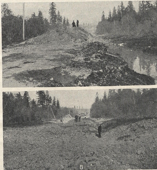
FIGURE 8.—A, OLD ROAD LOADED WITH BORROW MATERIAL BEFORE UNDERFILL BLASTING; B, THE SAME SECTION OF ROAD SHOWN IN A AFTER BLASTING. THE FILL MASS SETTLED APPROXIMATELY 15 FEET. NOTE THE SWAMP MUCK PUSHED OUT ON EACH SIDE.
