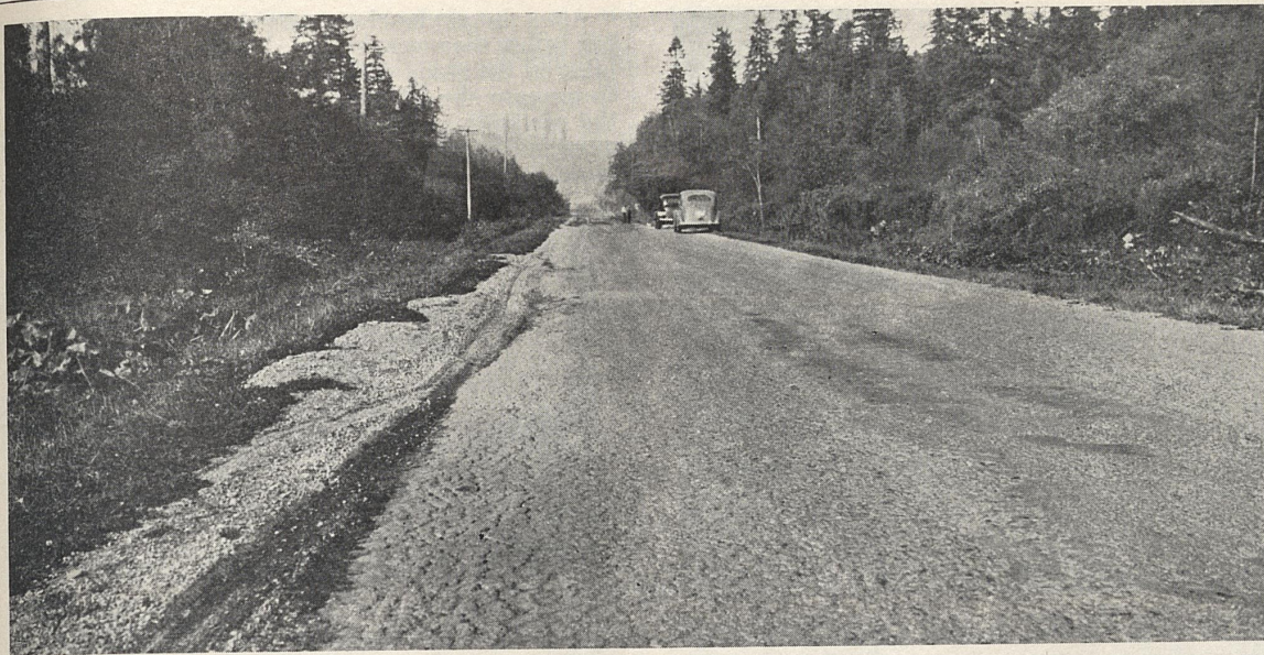
FIGURE 1.—EXISTING ROAD PRIOR TO RECONSTRUCTION. PICTURE TAKEN AT STATION 235, SHOWING CRACKS CAUSED BY UNSTABLE SUBGRADE.
