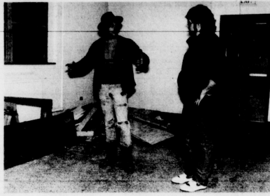
Alan Hawbe/Kernal Staff A Radio Free Lexington member looks over the construction of the group's new radio station, located in the Student Center.
