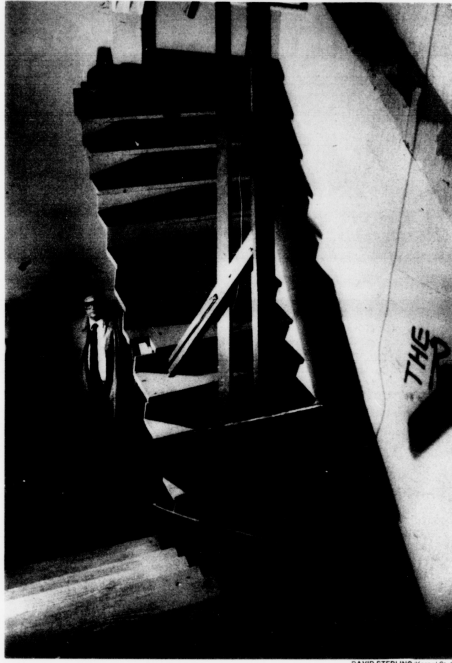
The staircase at the Reynolds Building collapsed yesterday, injuring five students. DAVID STERLING/Kentucky Staff
