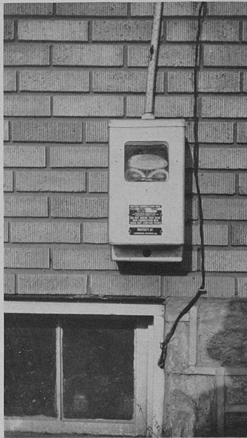
FIGURE 4. Watt-hour meter housed in weather-proof metal box.
