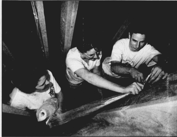
HANGIN' AROUND THE HOUSE UK students Jera Utley, Chris Manning and Brent Cox hang plastic over insulation in a Habitat for Humanity house being built on Dunaway Street.
