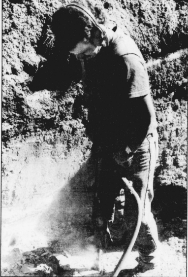
ON THE MOVE Charles Rose (above) is working on the renovations at Shawneetown. Resident David Schoenbacher (far left) looks on.
