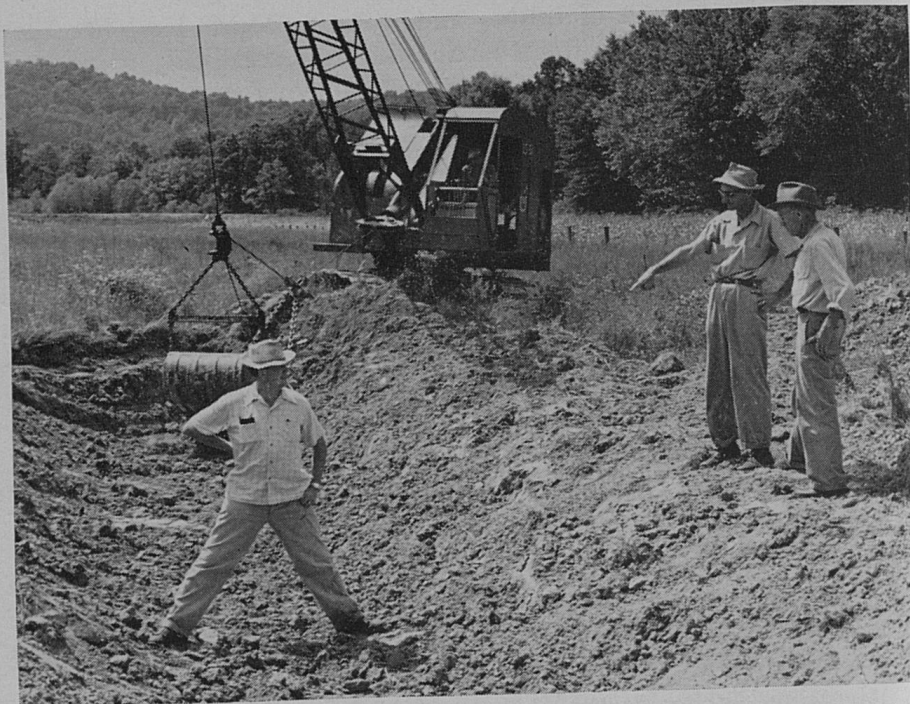
Bottomland pastures often require open ditches for surface drainage during rainy periods.
