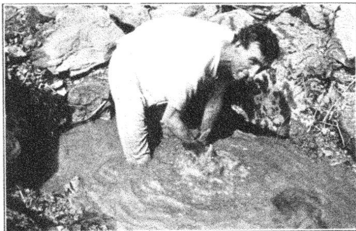
NOT BATHING—REPAIRING A LEAK
