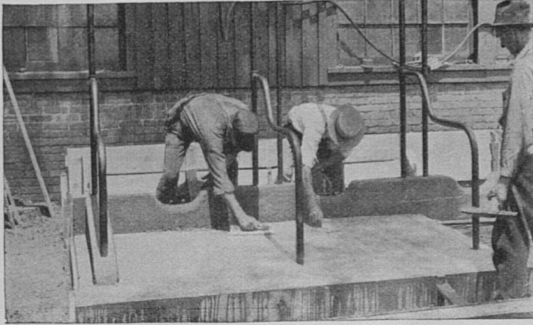
Fig. IX. The men are finishing the concrete stall platform with a wooden float thus giving it a rough surface.
