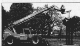
PHOTO BY CHLOE HOLLON / STAFF A crane installs a new art installation in the UK Art Museum sculpture garden on Monday. The sculpture parallels Africa's and Kentucky's dependence on coal.
