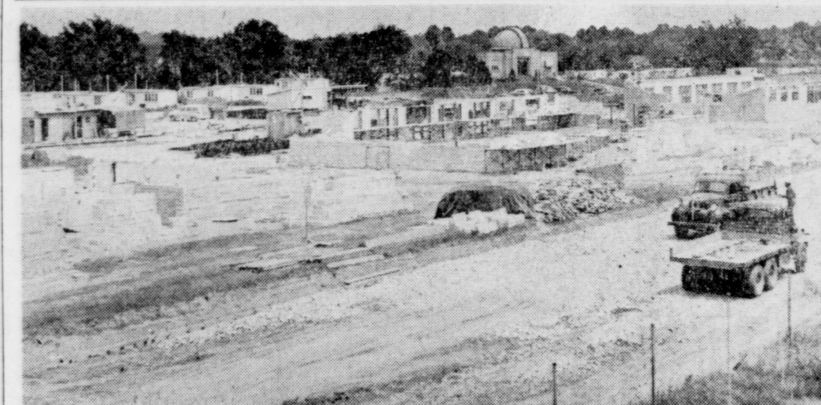
CHRISTMAS GIFT — Work on "fraternity row" is progressing rapidly. The contractor expects to have the six buildings ready by Christmas and the fraternities are scheduled to move in before the January semester. The fraternities which will move in are Sigma Chi, Phi Sigma Kappa, Lambda Chi Alpha, Kappa Sigma, and Pi Kappa Alpha. The sixth building will probably be used as a graduate men's dormitory.
