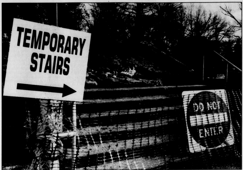
Construction junction The stairway across South Limestone Street is being repaired. A sign directs students to an alternative route to get to Dickey Hall and the Taylor Education Building.
