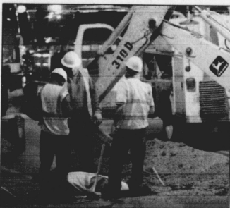
Workers from Columbia Gas Company dig up Rose Street last night after a gas leak was detected. Rose Street was closed for approximately three hours while the broken line was replaced.
